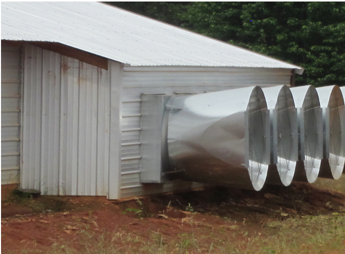
E. Tunnel fan light trap false wall installed in a vestibule plenum (dog house) in front of tunnel fans installed on the sides of the house.
