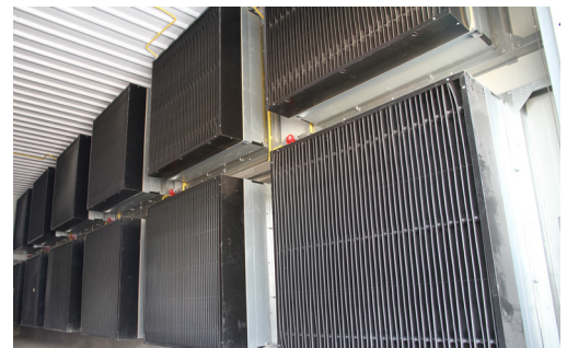
B. Light traps mounted over fans can reduce fan performance, and are not the best option in high-speed tunnel houses.
