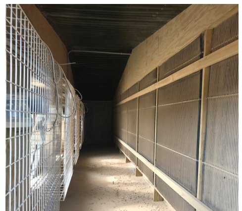
D. Light trap in a false wall in front of tunnel fans.
