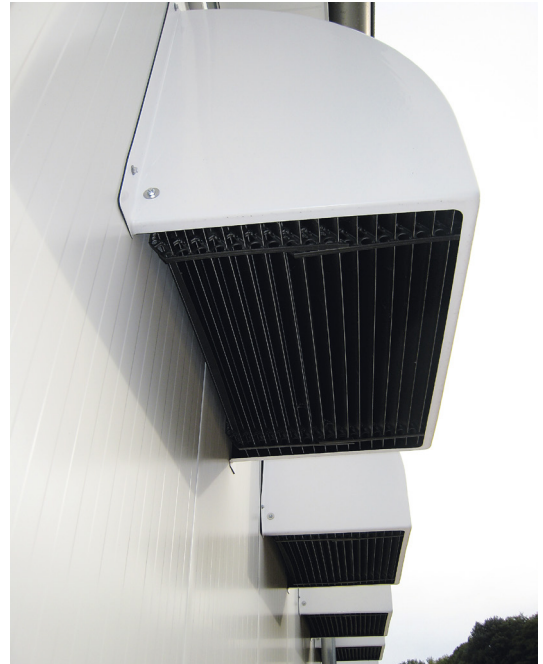
F. A perimeter inlet light traps installed in a box or wind proof cover.
